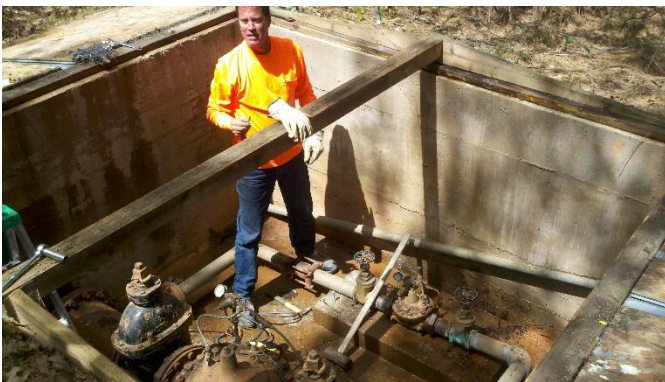
Left side: Rob working on one of the District's irrigation pressure stations.
